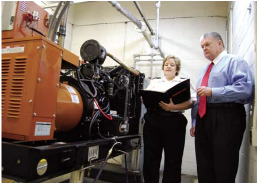
Captain Anna Cox, Commander of Communications & 911 goes over operations of the SJBPSO's new backup generator with Sheriff Jones.
